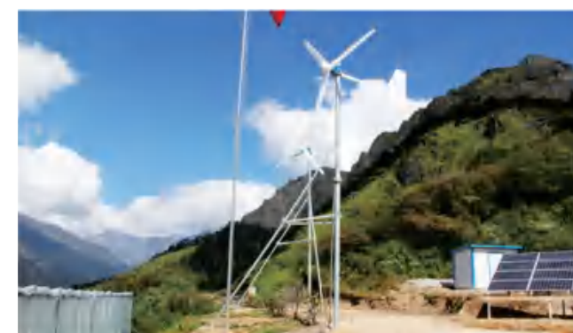
Model: FD5-5 Project location: Xizang municipality Run time: 2009 Project description: The base station is 5600 meters above sea level, and the lowest temperature is -40 Celsius degrees.
