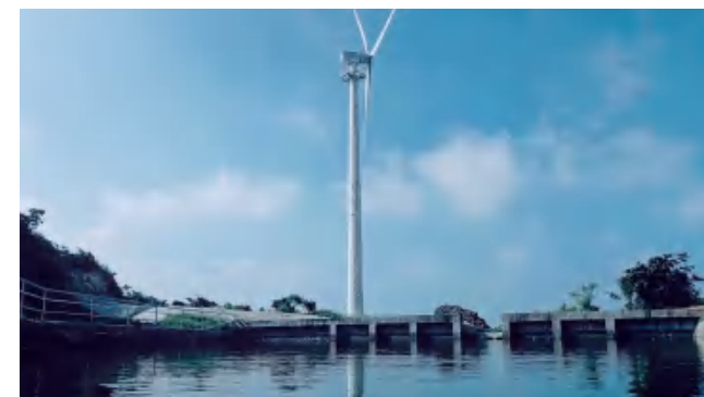
Model: FD5-5 Project location: Nomrog-united blinder Run time: 2010 Project description: Ghrepower and ZTE jointly built the site, Ghrepower is responsible for providing the wind turbine and control system, set up 13 sites in Mongolia
