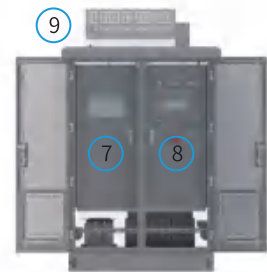
Figure 2 Inverter and Controller Integrated Cabinet
